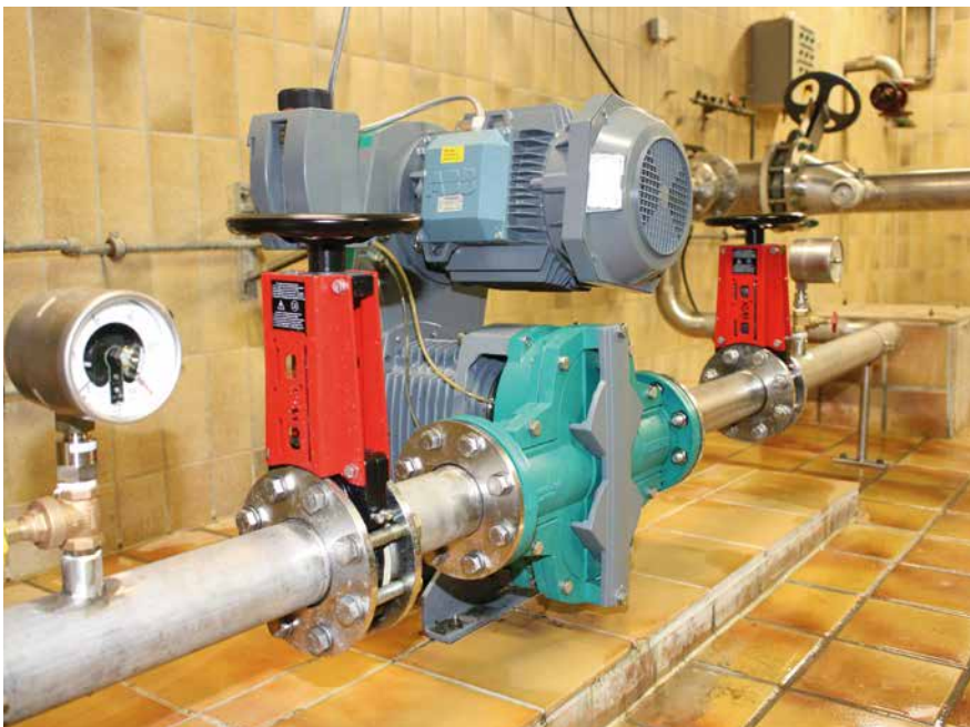
Centrifuge feed: 2 % DS excess sludge at a flowrate of 18 m 3 /h against a discharge pressure of 1,5 bar.
