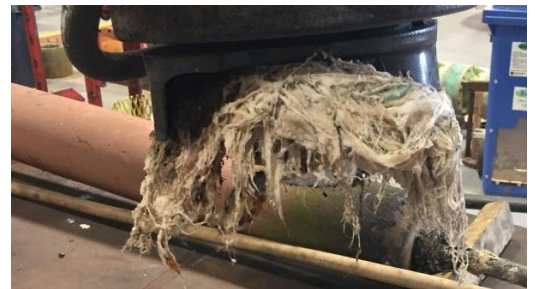
Above: Blockage materials entering the pump.
