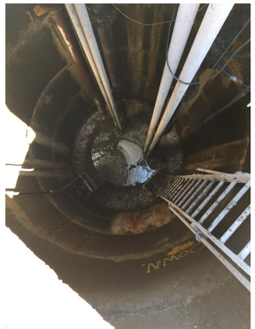
Above: Clean wet well at Butterknowle Green Sewage Pumping Station.
